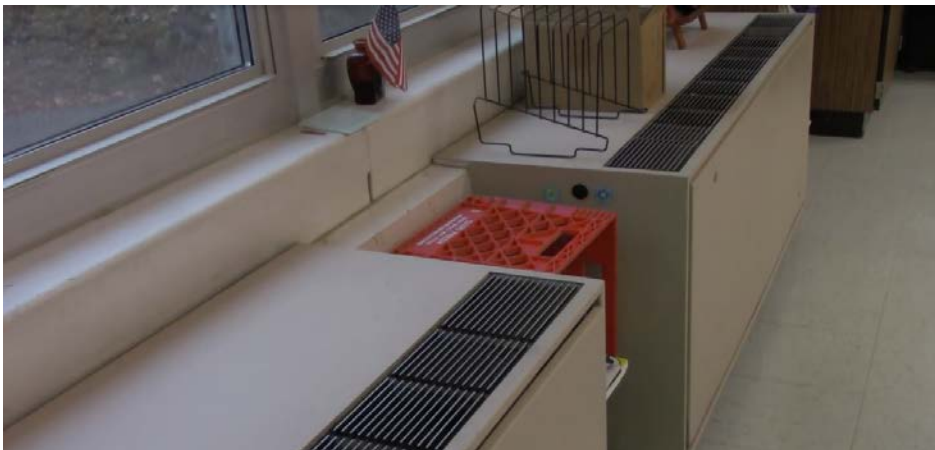
HVAC units in classroom
