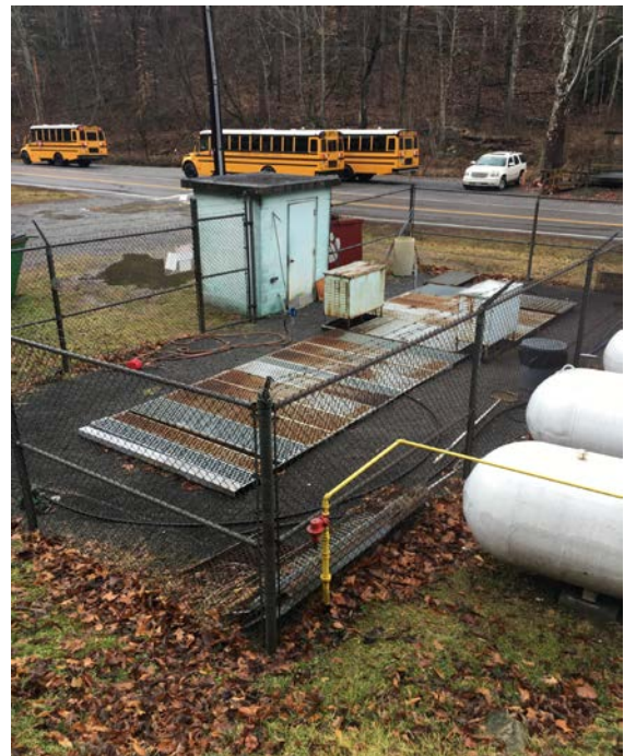
Wastewater treatment plant
